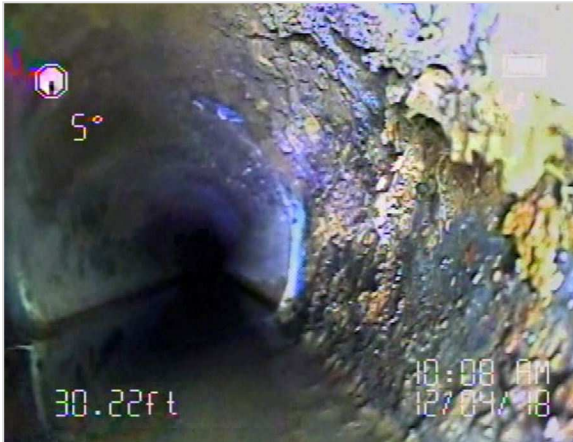
Transition to PVC – Standing Water - ~31ft
