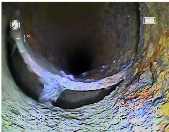
Pipes Separated - ~18ft
