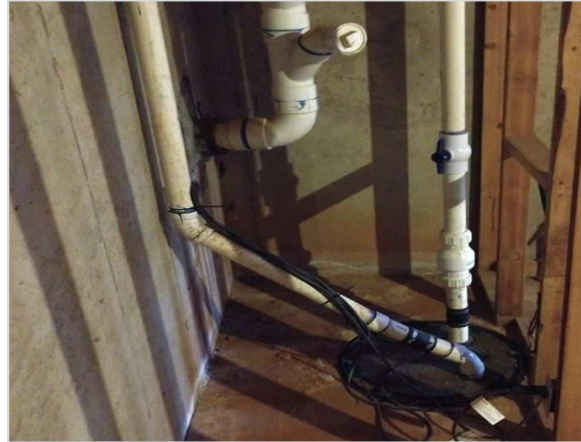
Cleanout in Basement
