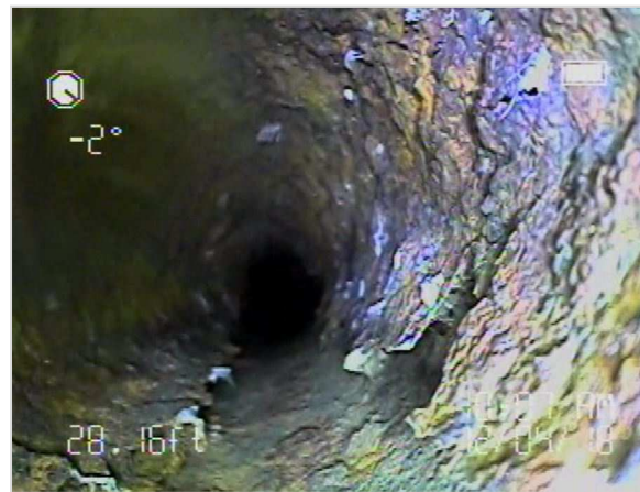
Cast-Iron – Poor Condition - ~28ft
