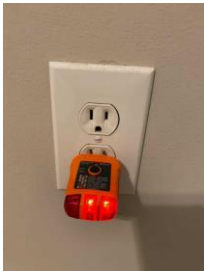
18. Acceptable HVAC Source: Heating system register
